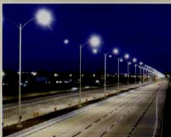
ELECTRICITY & STREET LIGHT
